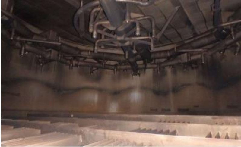
Figure 20. Interior of a scrubber tower with nozzles and demister.
