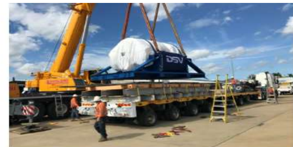
The transformer has safely arrived in Australia.
