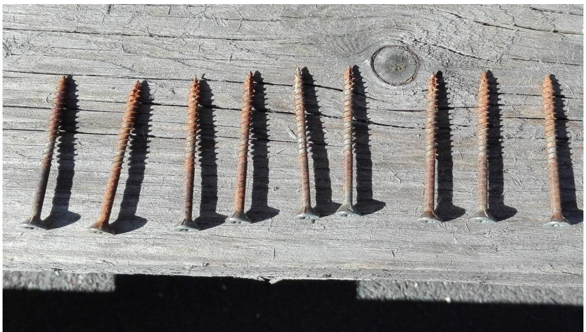
Figure 23. Galvanized screws removed from performance table on 5 th of May 2017 for inspection
