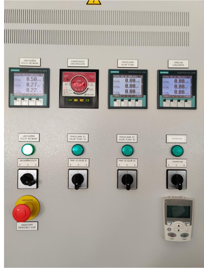
Microgrid main electrical panel; PAC3200 power metering devices
