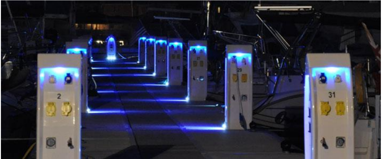
Figure 2: Rolec Spinnaker service pedestals at night. Source: Rolec Ltd
