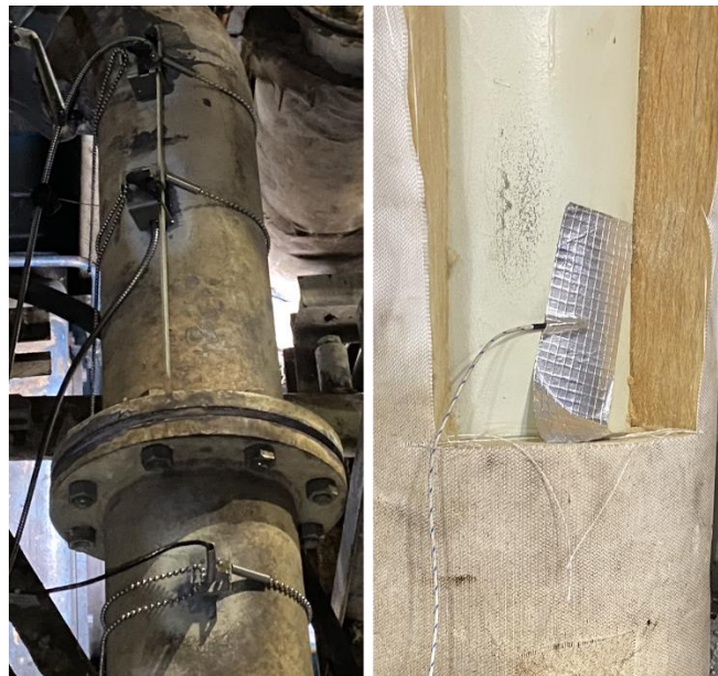
Figure 3.6 The main engine's HT cooling water measurement, FM and TT on the left, TL on the right
