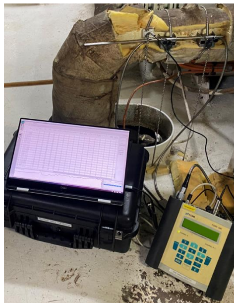
Figure 3.8 The boiler's feed water flow measurement, FM and TT
