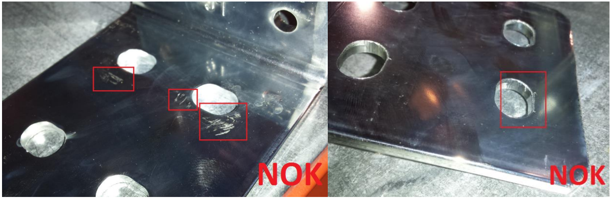
Figure 7.15. Picture of the former „as-is“ situation with busbars with sharp edges (NOK)
