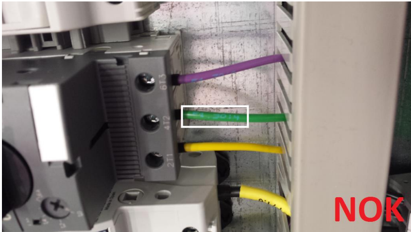
Figure 7.13. Picture of the former „as-is“ situation with wires with poor markings (NOK)
