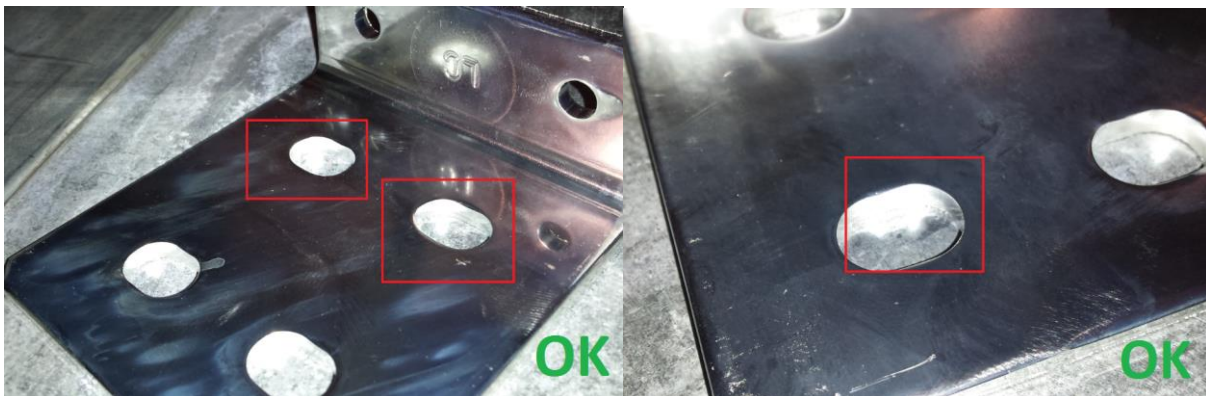
Figure 7.17. Picture of the improvement – sharp edges removed from busbars (OK)
