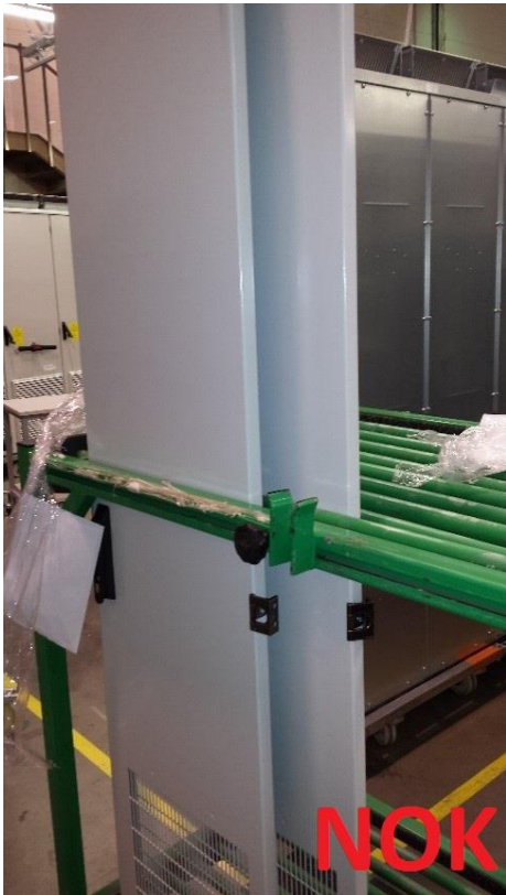
Figure 7.20. Picture of the former „as-is“ situation with danger of doors getting mechanically damaged (NOK)
