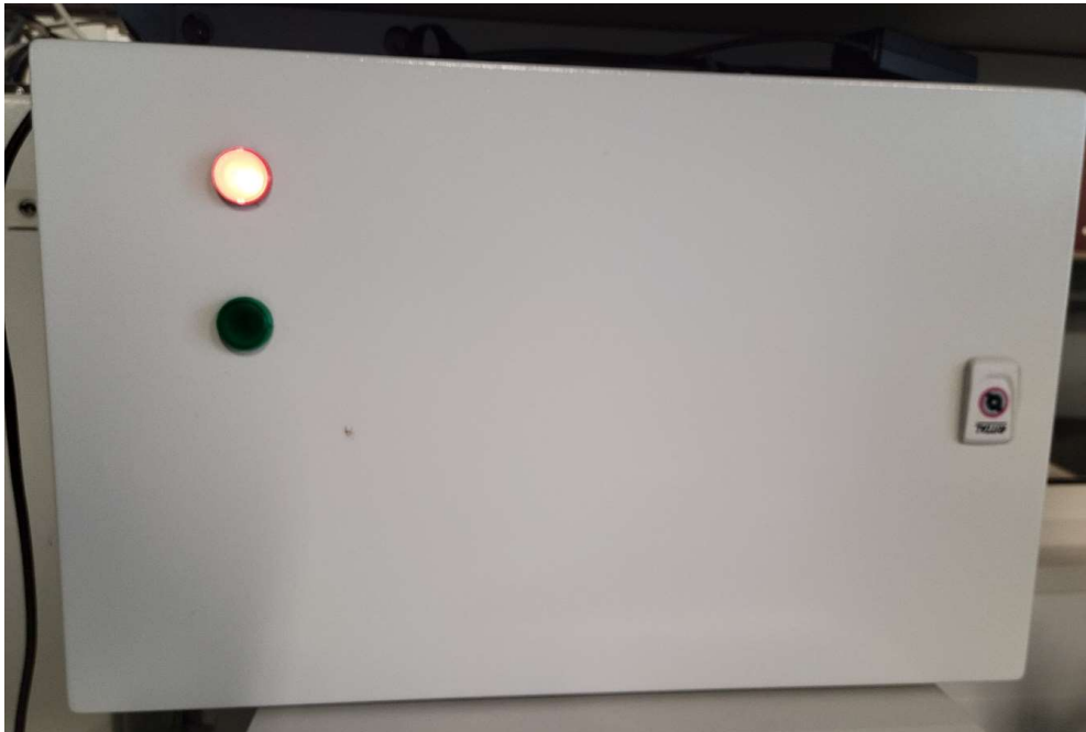
Figure 13: Control cabinet alarm lights
