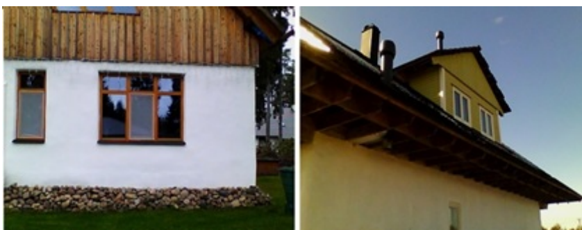
Figure 4. The examples of the plinths (left image) and eaves (right image) of the studied buildings. (Raamets et al., 2020)
