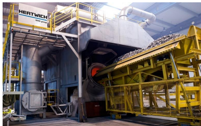
Figure 7. Rotary furnace at Herwick AB in work
