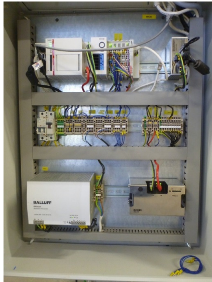
Figure 14. Main control electrical cabinet.
