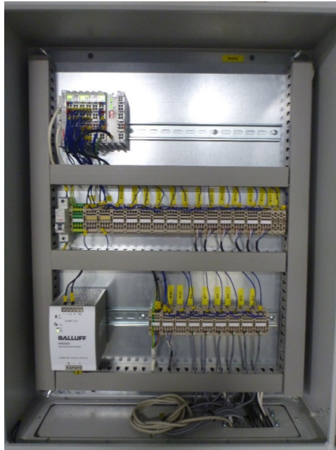
Figure 16. Remote IO electrical cabinet.
