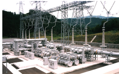
Figure 5: Gas insulated substation [19]
