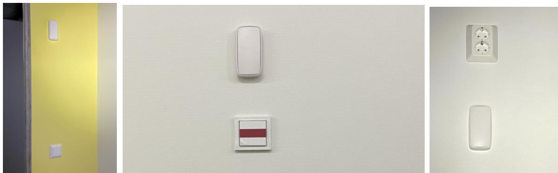
Figure 31 Photos of sensor installation
