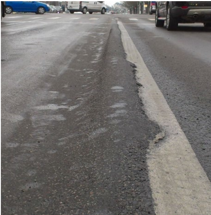
Figure 1. Extreme case of asphalt rutting on road nr E67 (Pärnu bypass). Rutting occurred soon after paving in summer 2012.
