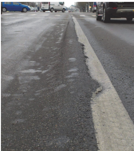
Figure 1. Extreme case of asphalt rutting on E67 Pärnu bypass. Rutting occurred on completely new asphalt pavement soon after paving in summer 2012
