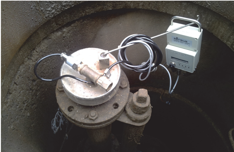
Figure 2-8 Pressure measurement solution at underground hydrant
