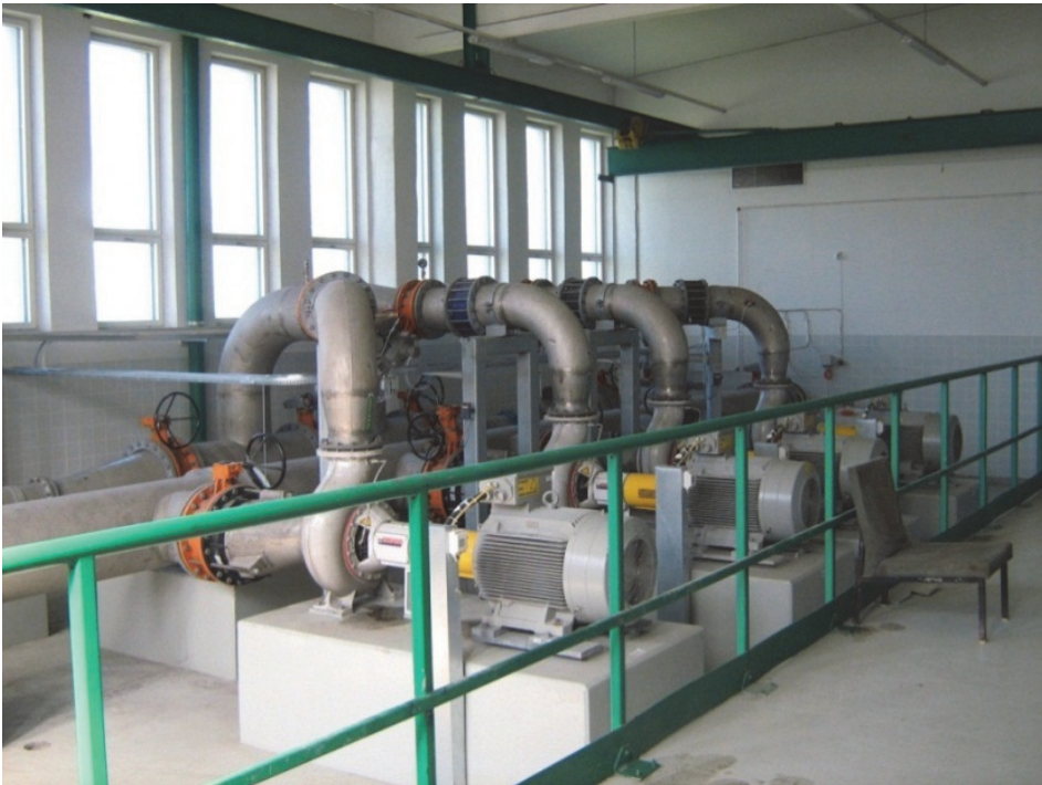
Figure 3-4 Inside view of the pumping station “Punane”
