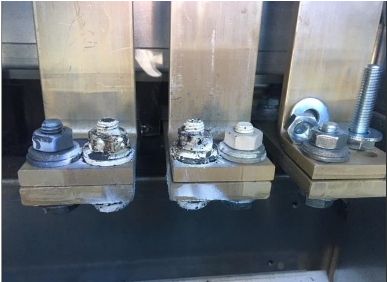
Figure 2. Burned connections on bus bars
