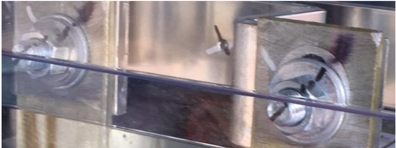
Figure 1. Loose connection caused by low tightening torque
