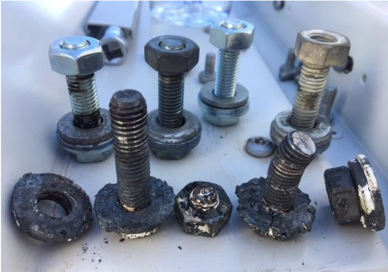
Figure 8. Damaged bolts and nuts
