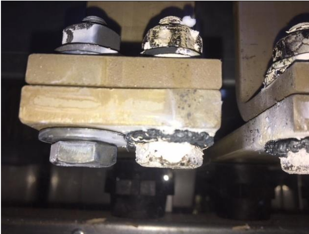
Figure 5. Damaged connection on first phase
