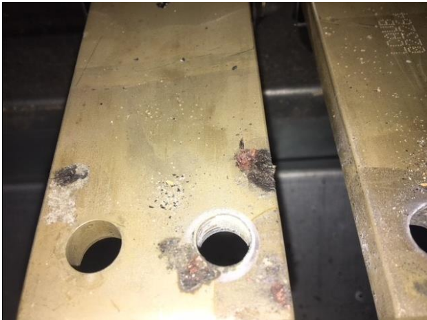
Figure 6. Arcing footprints on first phase bus bar
