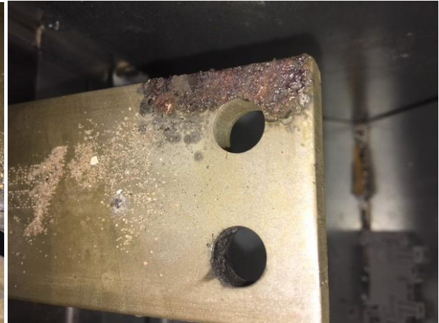
Figure 7. Arcing footprints on third phase bus bar
