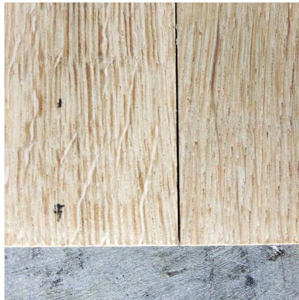
Figure 54. Crack along glue connection of boards.
