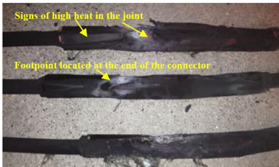
Figure 2.3. Faulty joint after separation of phases. [4]
