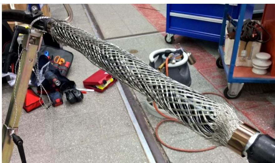
Figure 4.7. Aluminium sheath in the joint. The metal rings compress it onto the aluminium foil in the cable bulk.
