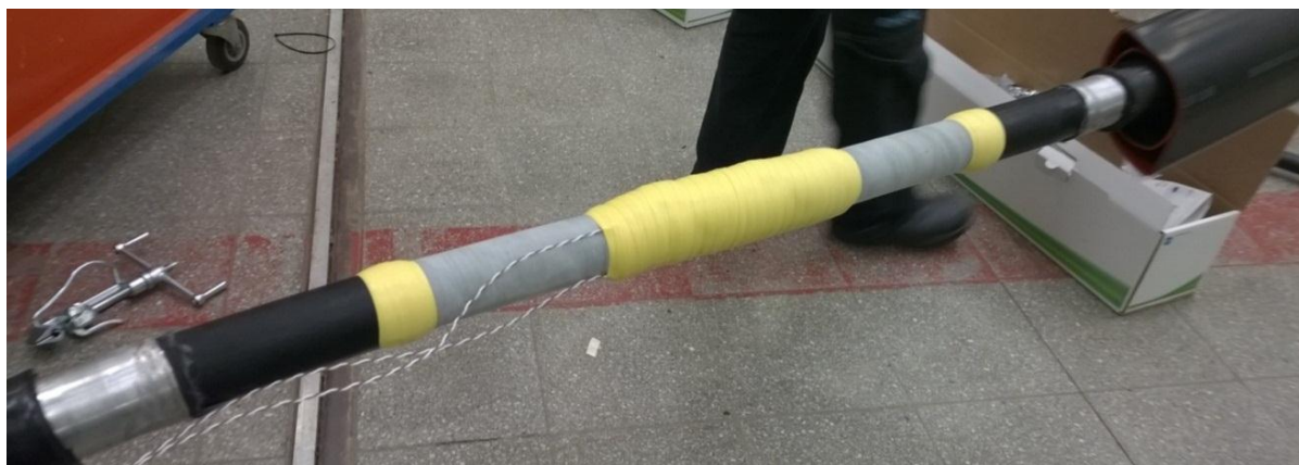
Figure 4.6. Field control tape on the connector. The insulating tubes (2 layers) are visible on the right side of the image.
