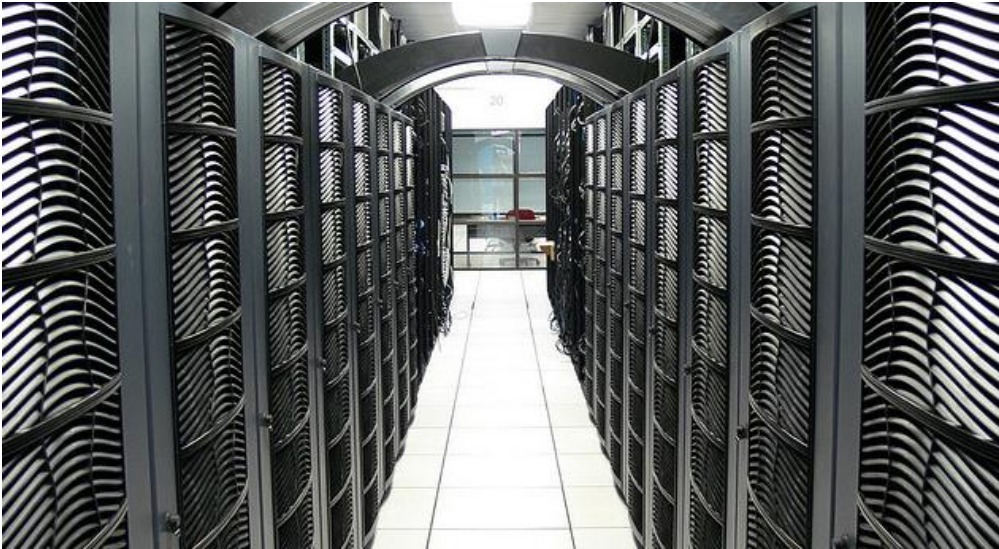
Figure [3] Data centre isle
