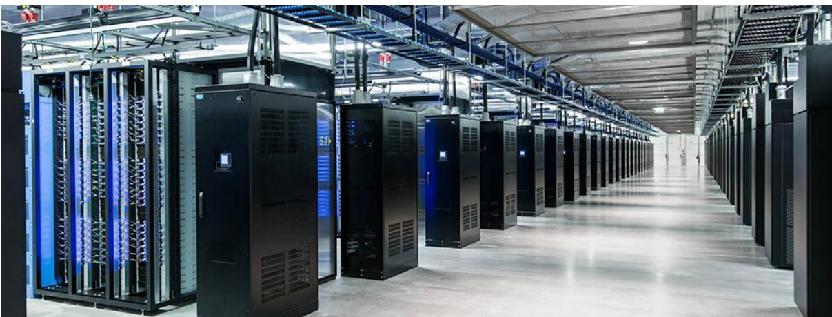
Figure [4] Facebook data centre in Sweden
