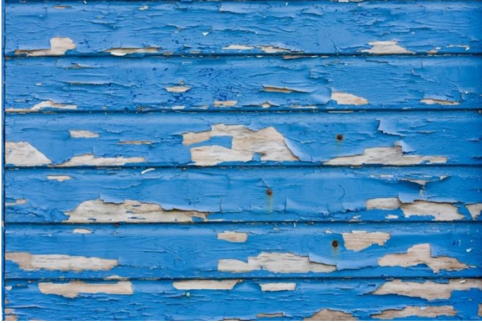
Figure 2.8. Flaking and peeling of the paint layer (Kaz, 2013)
