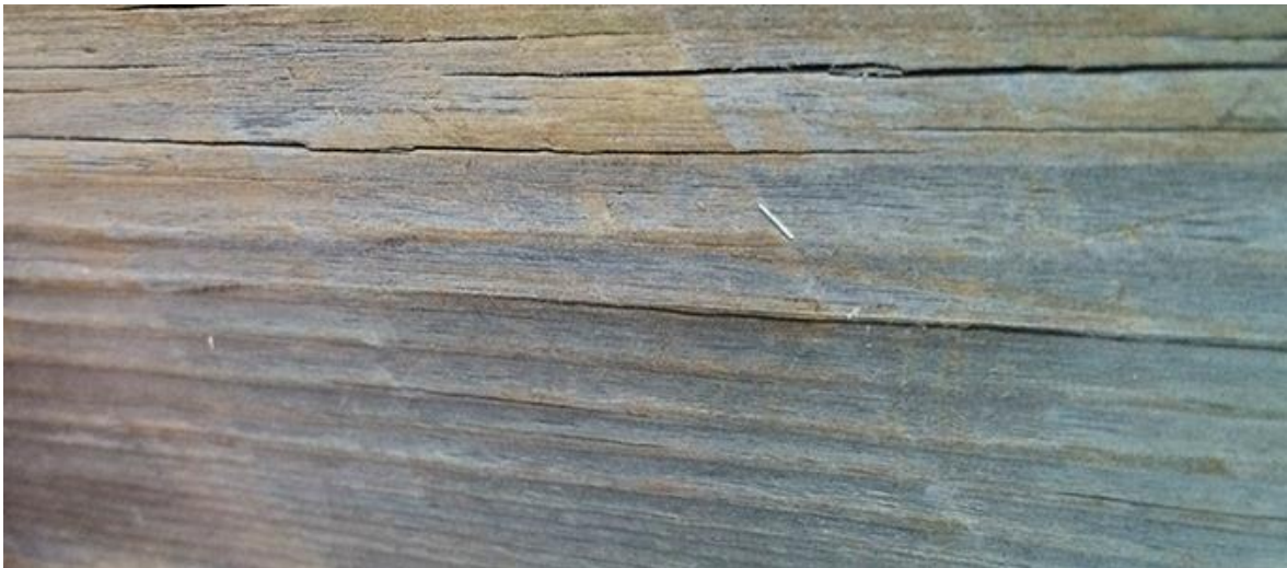
Figure 2.3. Checks on the weathered wood surface (GORI, 2017)
