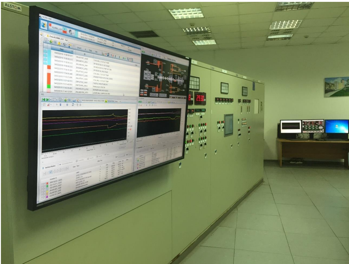
Figure 6. “Kosova B” power plant operational room [21]
