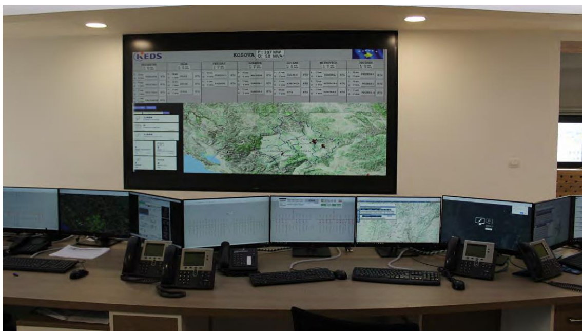
Figure 8. KEDS operational room where HMI of SCADA is shown [25]
