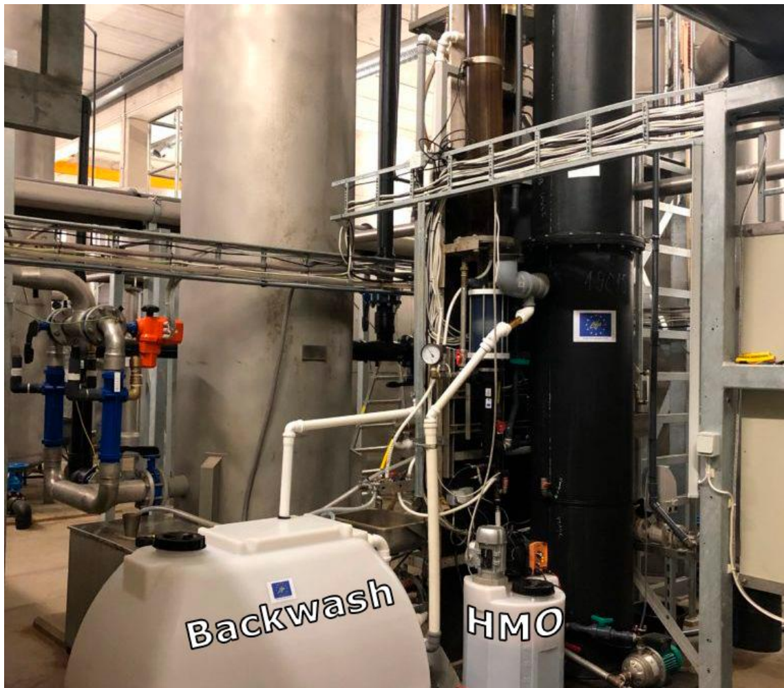
Figure 2.3 HMO tank and the backwash vessel near the contact column [30]
