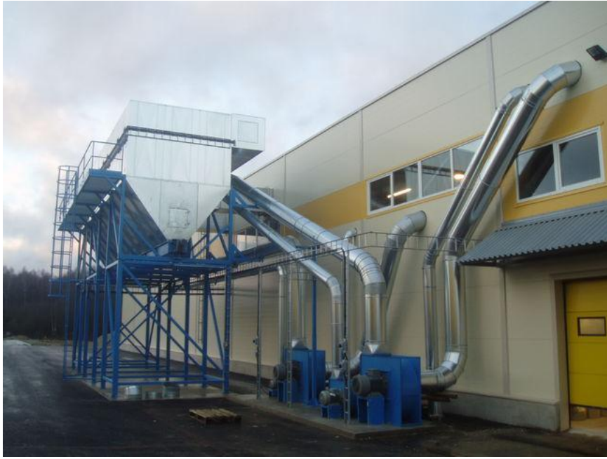
Figure 1.1 Hekotek recirculation filter [1]
