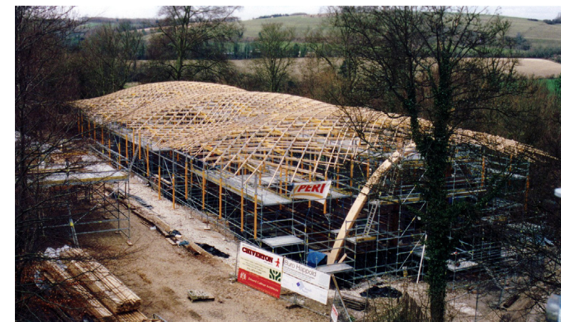
Figure 23. Construction of the Weald and Downland gridshell using PERI scaffolding. Source: Cullinan Studio
