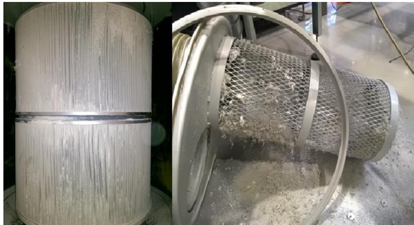
Figure 25: Dust removal system filters situation
