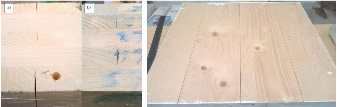
Fig 3. Cracks have been formed between laminations and in odd and even layers (left) as well between laminations over the entire length of panel (left) of S4.
