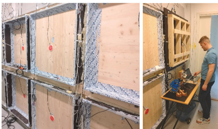
Fig. 2. CLT external test walls with the room view (left) and performing an air permeability test (right).
