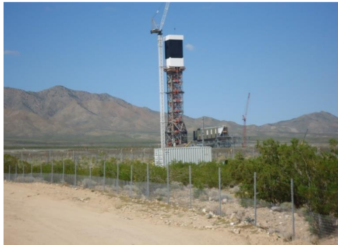
Figure 7. one of the three towers in Ivanpah power station Taken by author
