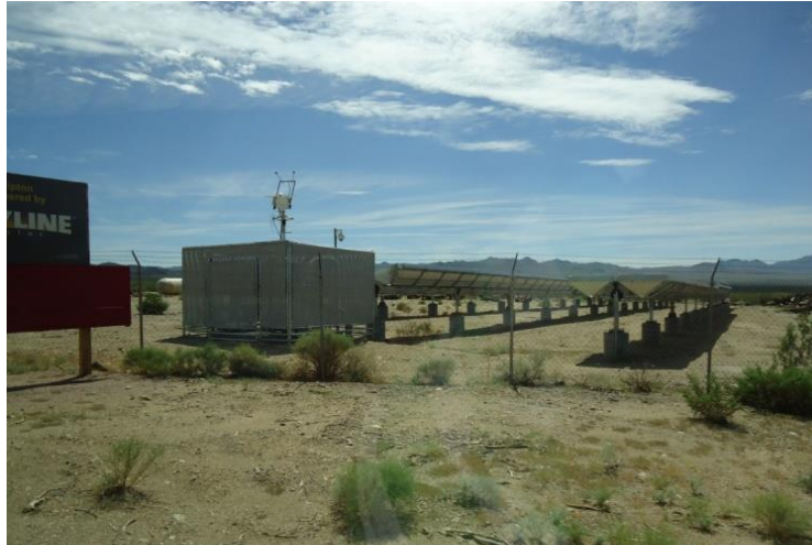
Figure 8. Nipton power plant. Taken by author
