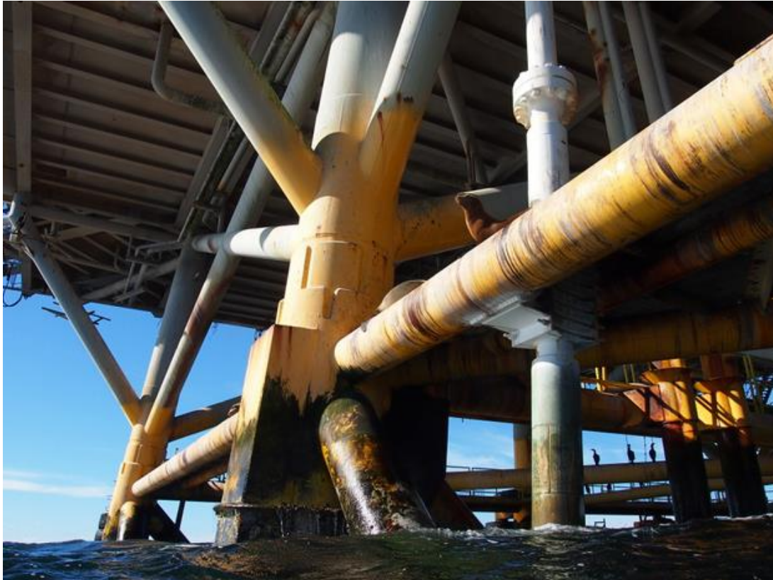
Figure 6. Close examination of the support joint on Eureka oil platform [2].
