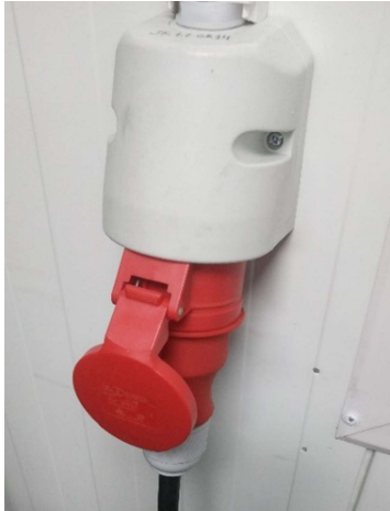
Figure 5 Power supply connected into wall socket
