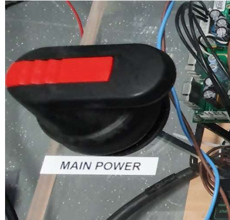
Figure 6 Main power switch
