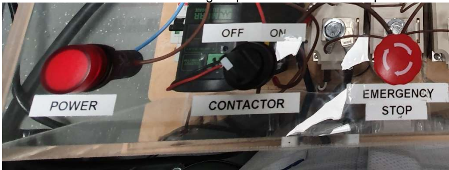
Figure 7 Contactor switch located in the middle
