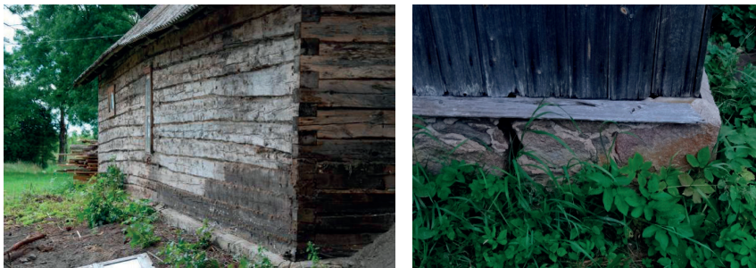
Figure 3: Uneven settlement of the foundation and an excessively low foundation wall (left) and cracks in the foundation due to the soil freezing and damaged water boarding (right).
