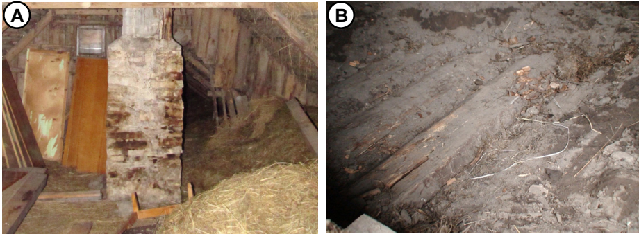
Figure 4.7. Fire risk in the attic (A). Rot damage to wooden ceiling details insulated with soil (B).
