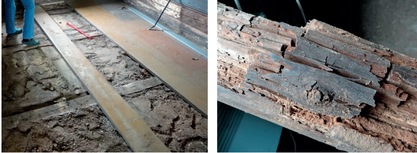
Figure 5: Floor beams inside damp soil (sand) (left). Floor planks are ~4 cm thick, and a ~1 cm thick layer from the lower surface is rotten (right).
