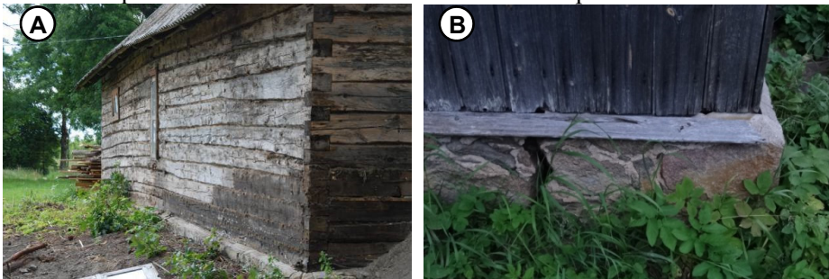
Figure 4.2. Uneven settlement of the foundation and an excessively low foundation wall (A) and large cracks in the foundation due to the soil freezing and damaged water boarding (B).
