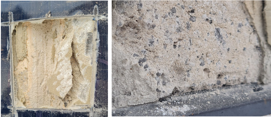
Figure 40. Discolouration of the PCM mortar (slightly orange surface to the left of the diffusion channel) (left). Structure of the PCM mortar after full removal of the PV panel (dark grey particles are PCM granules coated with PU, colour of the mortar is uniformly light grey both near the granules and further away) (right).
