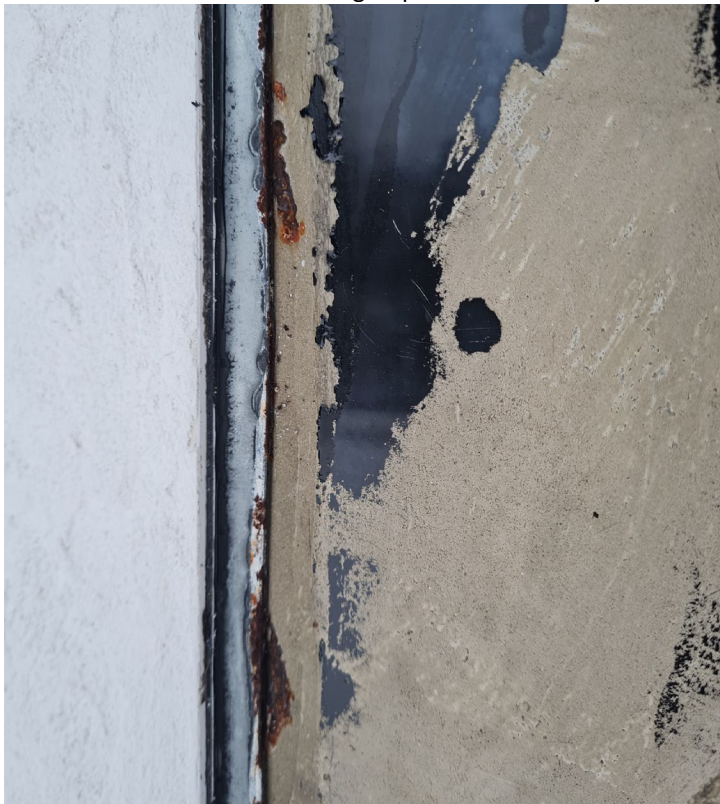
Figure A7.3. Signs of corrosion on the zinc-coated steel sheet ribbon after removal of the PV panel on 10.02.2026.
