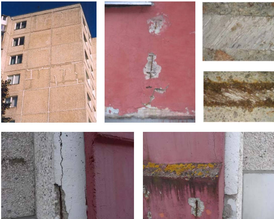
Figure 2.4. Reinforcement corrosion of the facade, top left and middle (private collection of Prof. Emer. Karl Öiger). Corrosion studied with microscope in laboratory – no corrosion yet, top right, and corroded reinforcement, middle right (Ilomets et al., 2011).
