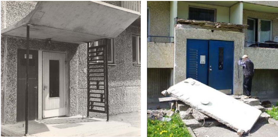
Figure 2.9. Reinforced concrete awning panel above an entrance door from the 1960s on the left (private collection of Prof. Emer. Karl Õiger) and a collapsed awning panel at Keila near Tallinn (Postimees, 2016).
