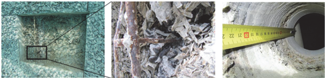
Figure 5 Reinforcement steel between layers of concrete has started to corrode (left and middle). In principle, this steel should be cast into expanded clay concrete, but in reality it is often not so. Cross-section of a concrete wall element (right).
