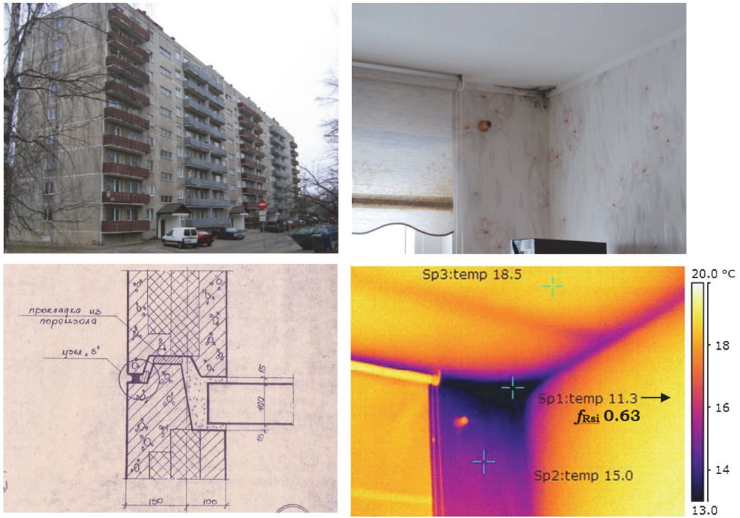
Fig. 4 Example of a precast concrete large-panel apartment building (upper left) with discontinued insulation in the junction of the external wall and floor (lower left). Visible mould growth at the corners of a
