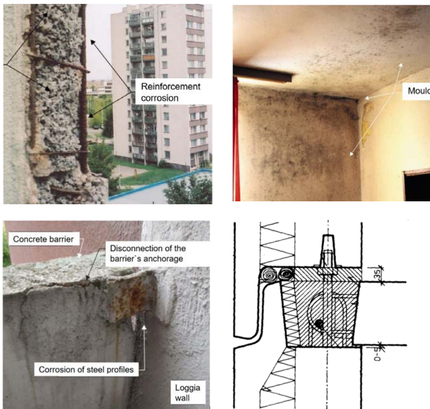
Figure 2.5. Extensive reinforcement corrosion and the concrete cover dropped off (top left) and extensive mould growth on the interior surface of the building envelope (top right). Corroded anchoring detail of the RC loggia barrier (bottom left) and a vertical junction of two external wall panels and the floor slab (bottom right), all from (Witzany, 2016).
