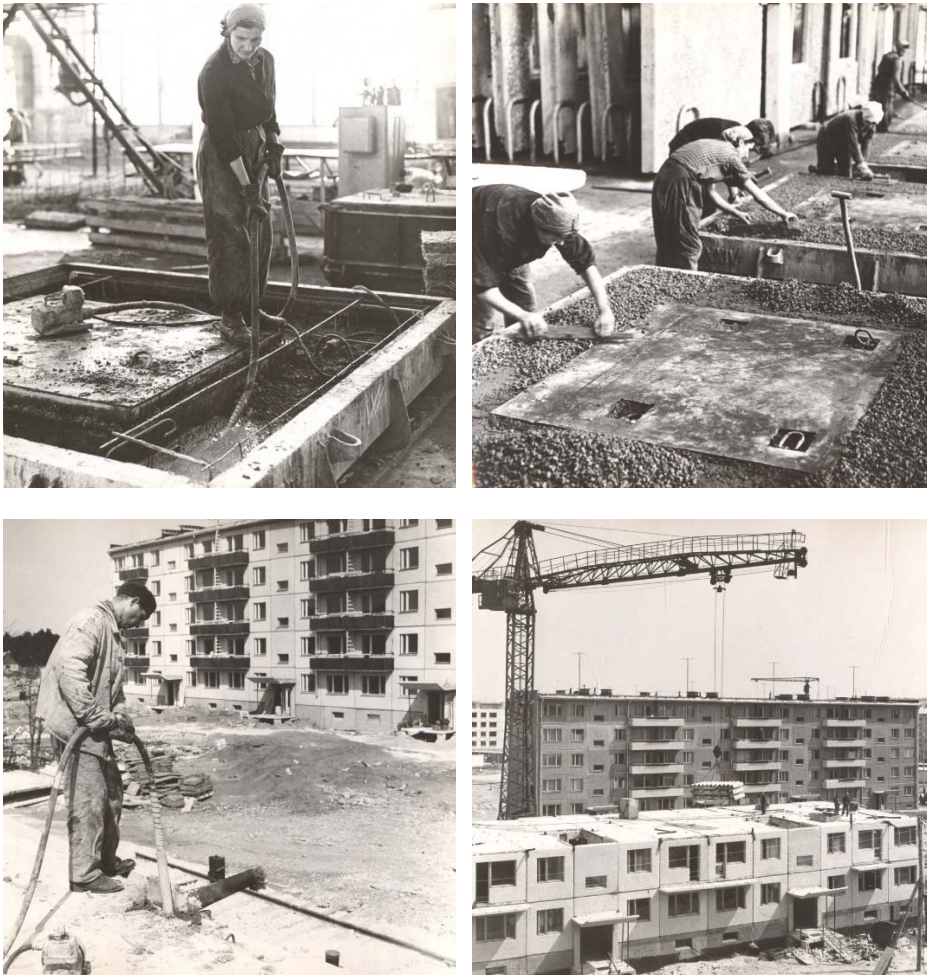
Figure 2.2. Casting the internal layer of concrete into the formwork with steel reinforcement (top left), levelling the rubble bulk of the incoming facade (top right), casting the concrete into the junction in situ (bottom, left) and mounting the panels by crane (bottom right), all from the private collection of Prof. Emer. Karl Öiger.
