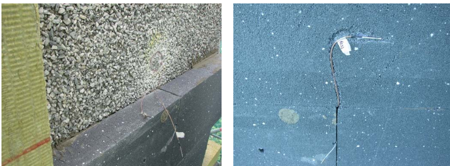
Figure 4.3. Illustration of the case study measurements: original reinforced concrete wall covered with rubble bulk and the wiring (left) and the temperature and relative humidity sensor (right).
