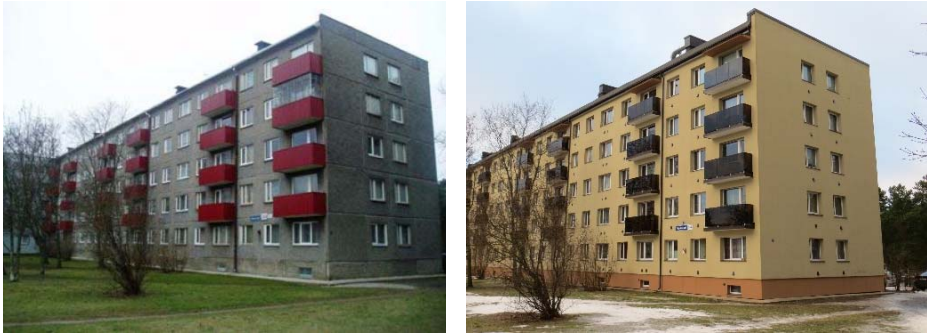
Figure 3.1. Reinforced concrete external wall of a case-study building before (left) and after (right) the external thermal insulation composite system was installed.
