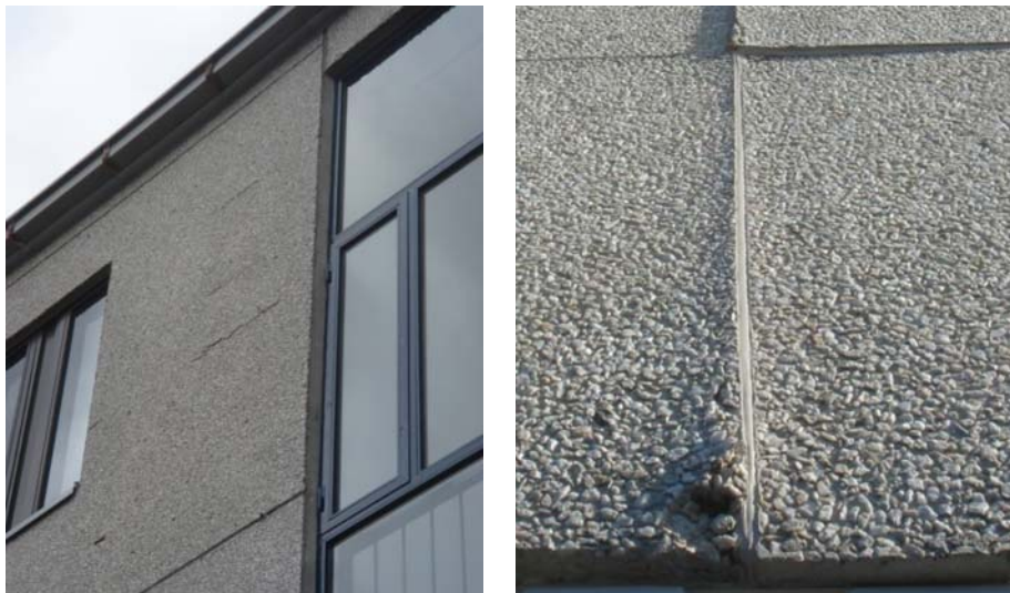
Figure 2.7. Typical carbonation induced corrosion on the left and local frost damage at the edge of an exposed aggregate RC panels on the right (Lahdensivu et al., 2013).
