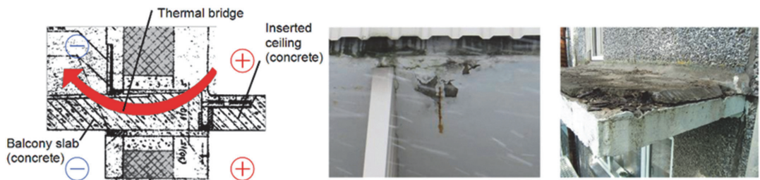
Figure 6 Original drawing of an external wall/console balcony junction with a thermal bridge (left) and a picture of a degrading balcony (middle and right).
