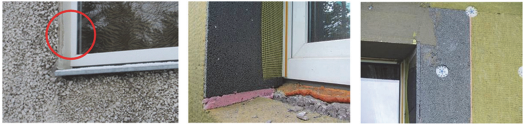
Figure 10 Picture of an old window (left) and of new windows placed at their original position. Most of the jamb is covered and only a thin layer of insulation (5...20 mm) can be attached to the jamb.
