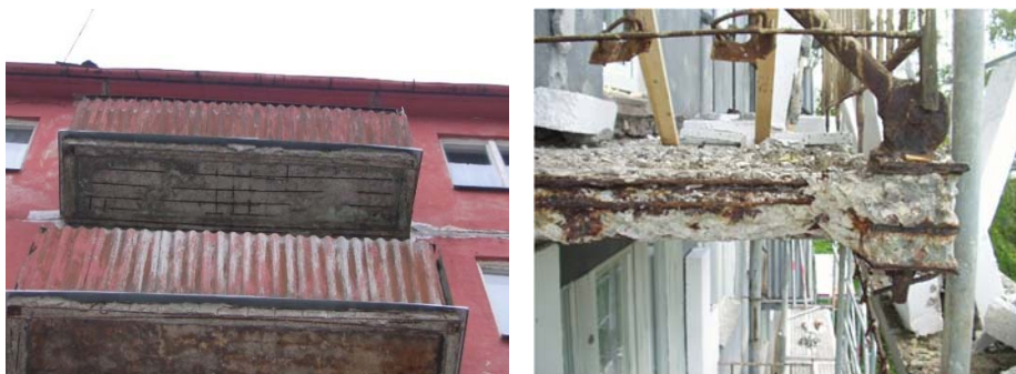
Figure 2.8. Severe corrosion propagation of reinforced concrete balconies (Õiger, 2006).
