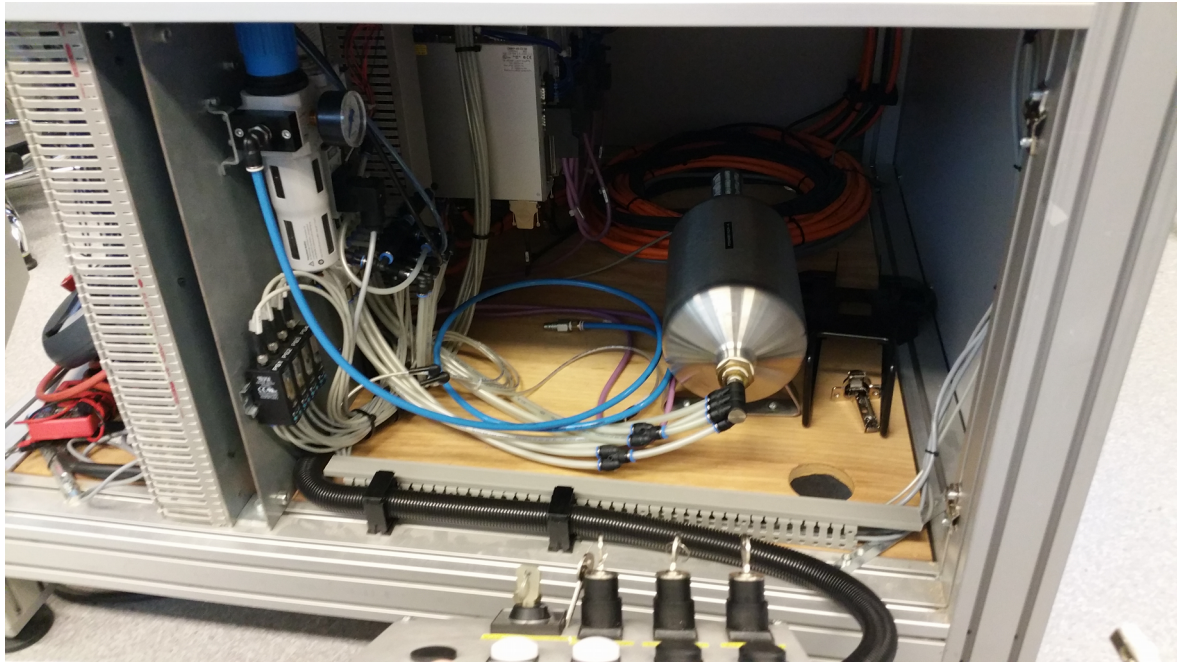
Figure 1.6. Drives and pneumatic compartment of the EXPT electrical cabinet.
