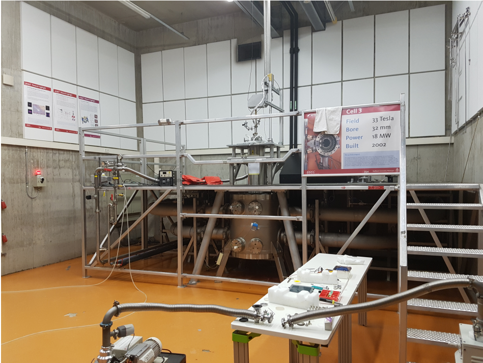
Figure 18: Nijmegen Bitter magnet setup at Cell 3. The Bitter magnet is at the centre of the picture under the platform. Four horizontal cooling water pipes are connected to the magnet, two from each side. Above the magnet from the level of the platform there is a cryostat, its tail extends into the 32 mm bore of the magnet. At the top there is a grey pipe, a part of the quasi-optical telescope, coming from the spectrometer that is situated on the upper floor. The two black vertical pipes at the back wall are the power cables. The red light on the left hand side wall shows that the magnet is currently under use.
