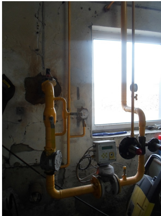
Figure 2.3 Natural gas supply point
