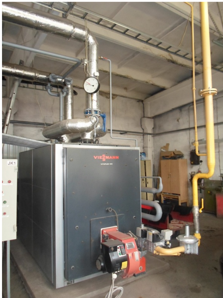
Figure 2.2 Water heat boiler Viessmann Vitoplex 100 1.12 MW
