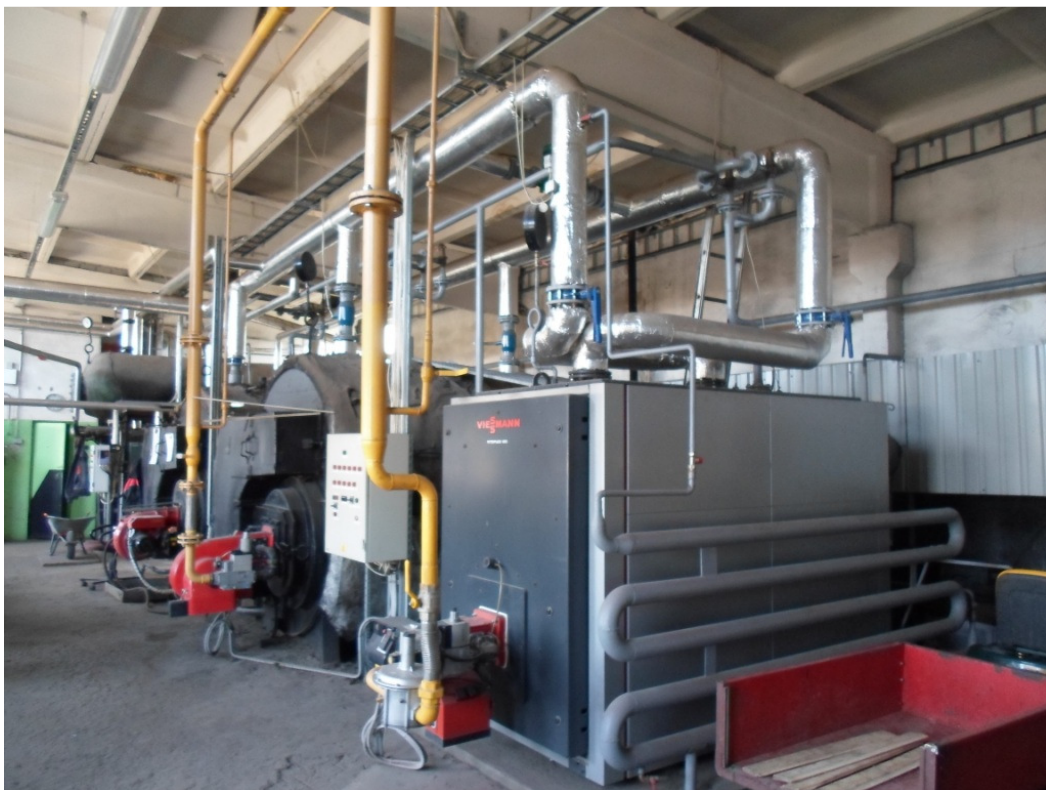
Figure 3.2 Olgina boiler house inside
