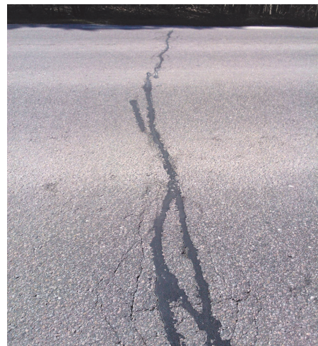
Figure 2. Typical pavement low temperature cracking with secondary fatigue cracking adjacent to transverse cracking
