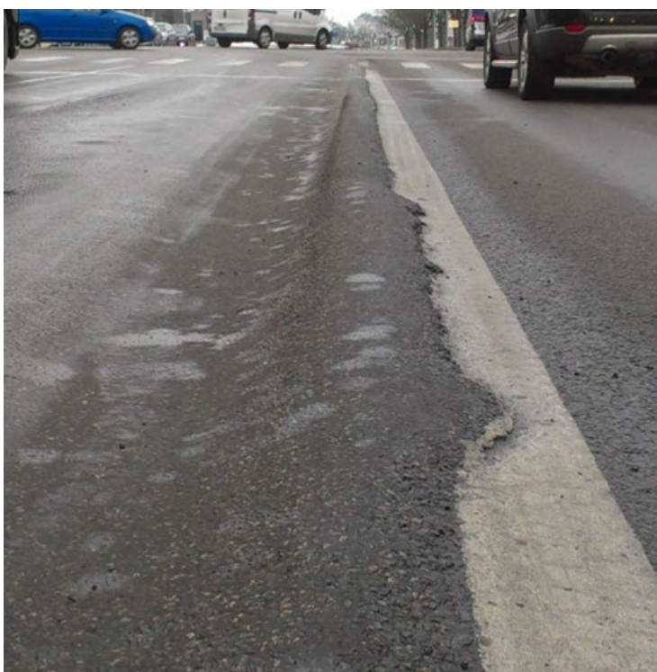
Figure 1. Extreme case of asphalt rutting on road nr E67 (Pärnu bypass). Rutting occurred soon after paving in summer 2012.
