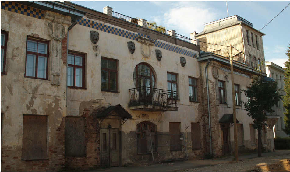
Figure 12. The cultural monument at J. Kuperjanovi 12 before restoration which will offer quality rental apartments for specialized labour force in the future (Valga municipality)
