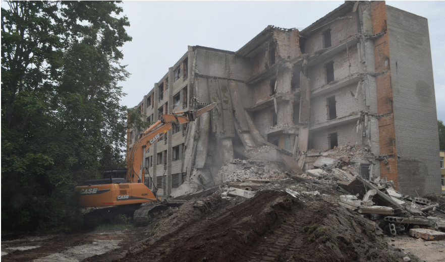
Figure 10. The demolition works of the former dormitory for railway workers (address Pikk 21A) in 2015 (Valga municipality)
