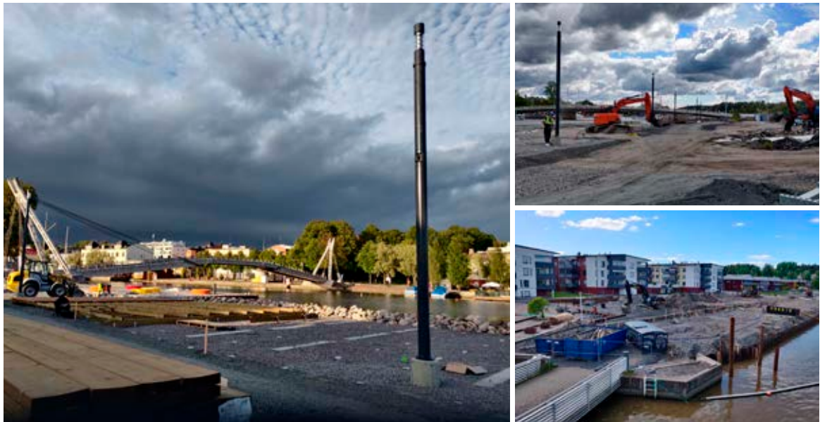
Figure 24. Construction works at the LUCIA pilot in Porvoo (all photos by Topi Haapanen).
