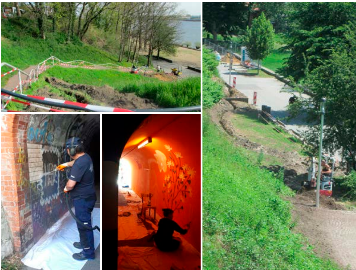
Figure 13. Construction and decoration work at the Hamburg pilot site (all photos by Bezirksamt Altona).
