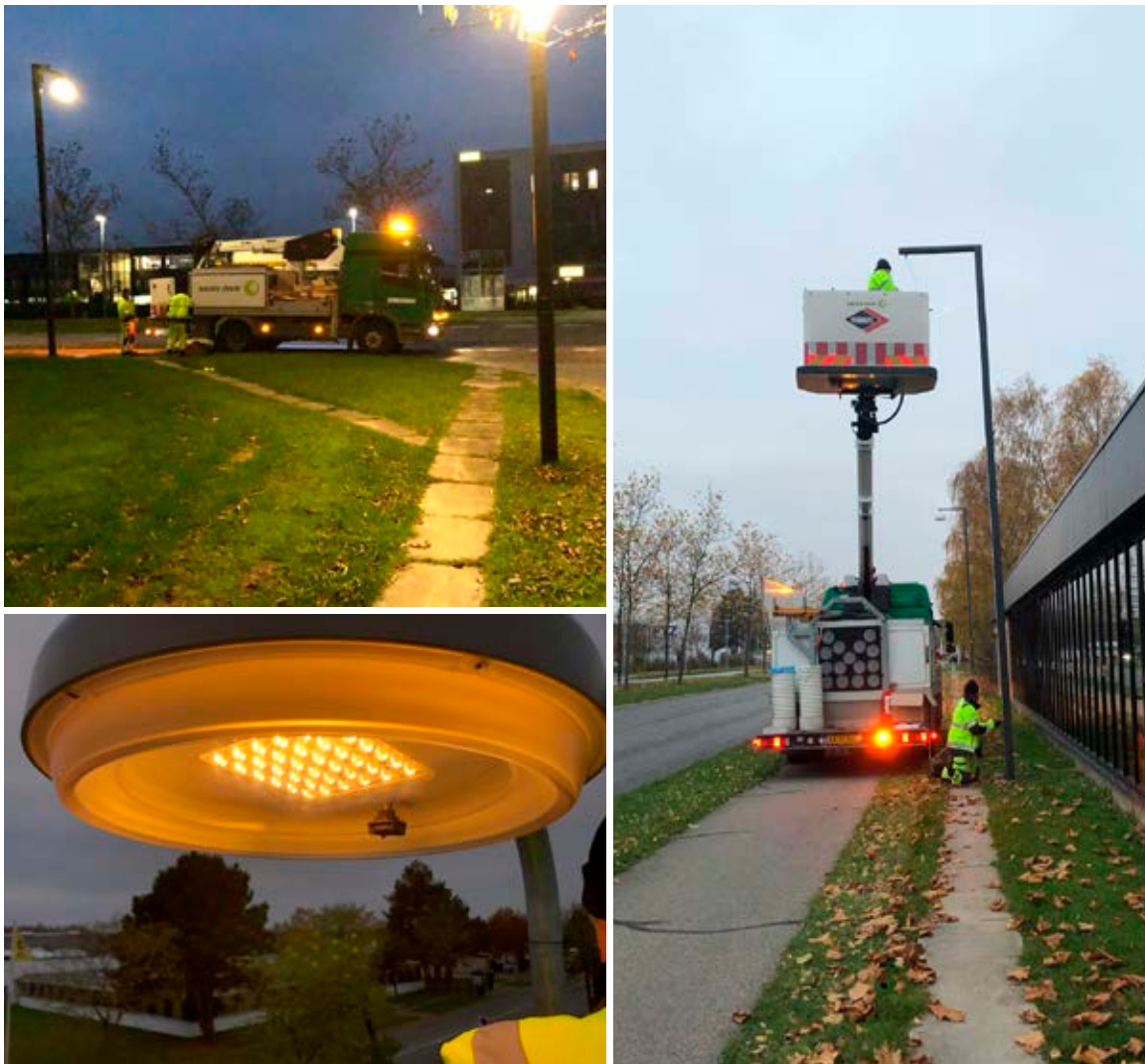
Figure 7. Installation works at the LUCIA pilot site in Albertslund (all photos provided by DOLL Living Lab).
