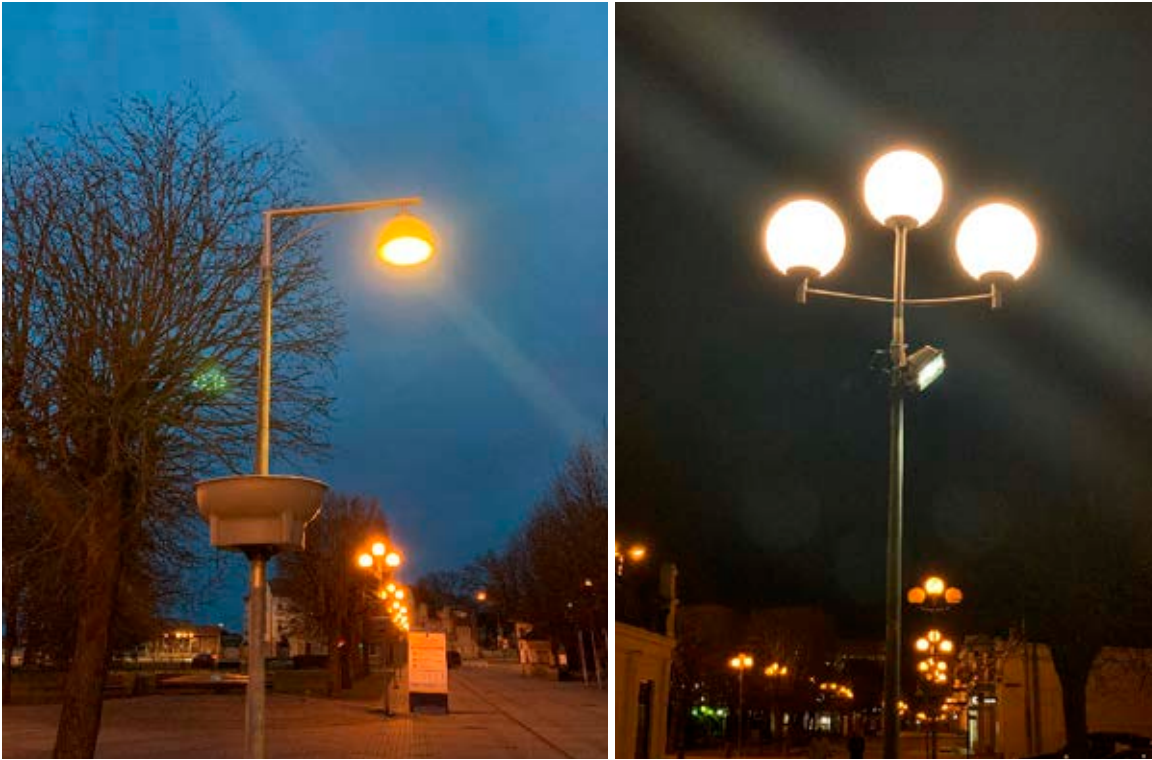
Figure 17. Before finalizing the technical design, different luminaires were installed and tested for initial verification (photos by Jurmala City Administration).
