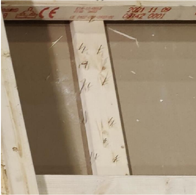
Figure 5.17 Staples missing the lath
