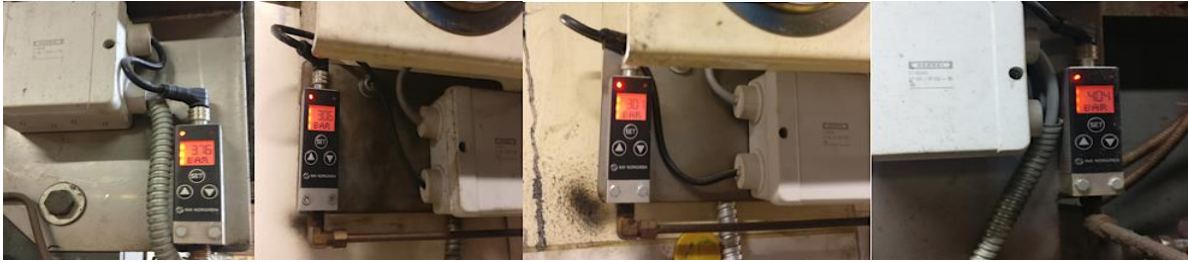
Figure 5.4 Pressure sensors on forming machines LPS feed pipes
