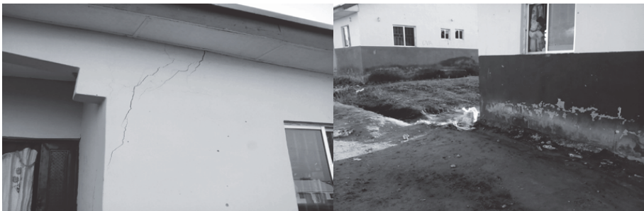
Figure 1(a) and (b) Figures showing visible defects on newly constructed houses for Post-2012 flood victims in Lokoja, Kogi State, Nigeria.
