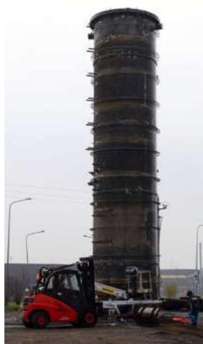
Chimney; weight 25.5t; length 37m; diameter 1.9m
