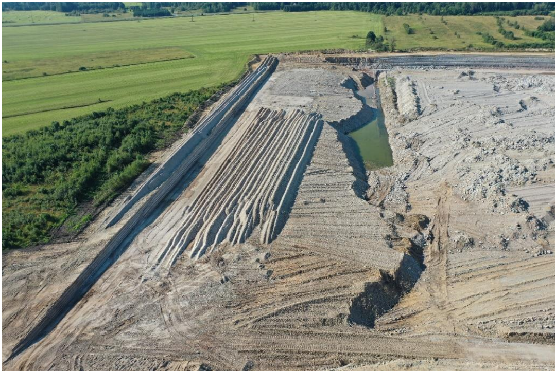
Figure 6. Aerial view of the chosen study area in the south-eastern part of the mine. (author's photo)
