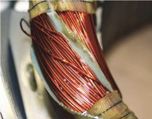
Fig. 4. Improper winding placement in Motor 3.
