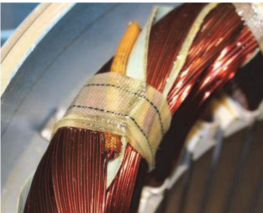
Fig. 6. Wire concatenation in the motor's winding in Motor 5.
