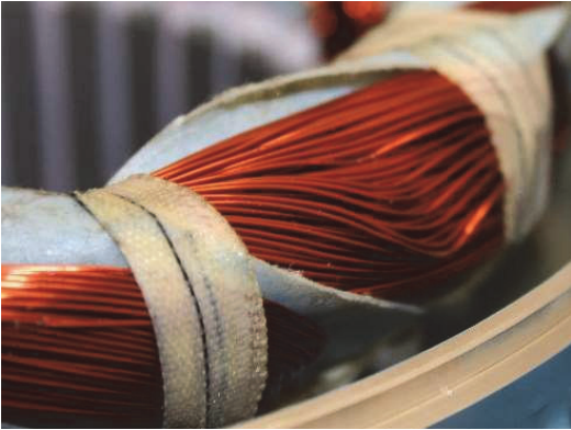
Fig. 10. Bruised winding in Motor 8.
