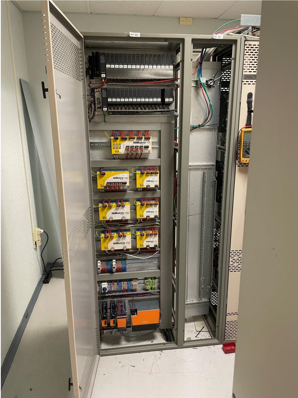
Figure 22 Water Heating Boiler 2 Cabinet Front
