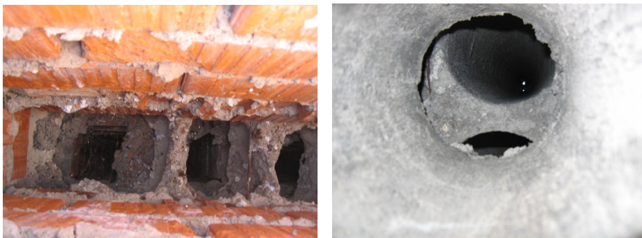
Figure 4. The installation quality of old ventilation shafts is poor (left and right).
