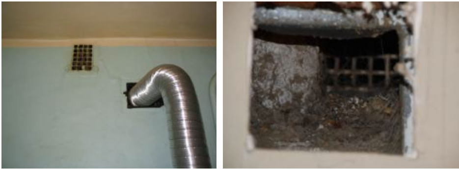
Figure 5. The connection between the old ventilation channels and ductworks of the kitchen hood are not airtight (left) and the dust have accumulated inside the old NV systems (right).
