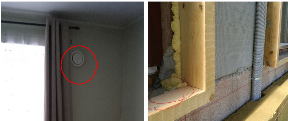
Figure 48. Supply air valve installed without sector plate (left) and apartment ventilation duct inside the insulation layer (right).
