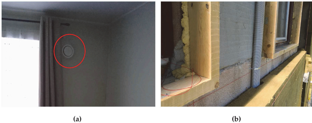
Fig. 13. (a) Supply air valve installed without sector plate and flat ventilation duct inside the insulation layer and (b) ventilation ducts inside the insulation layer.
