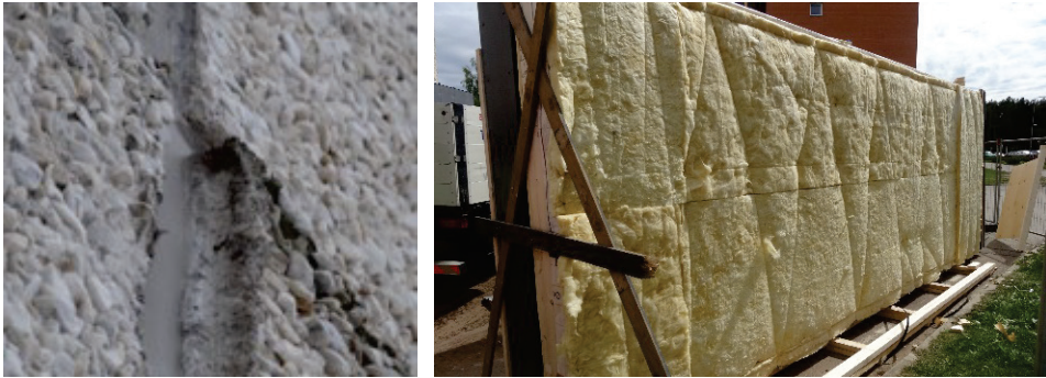
Figure 4.16 The original PCLP wall surface was rough and uneven (left). To smooth the surface, a buffering layer was attached on the back side of the prefabricated insulation elements (right) (2017).
