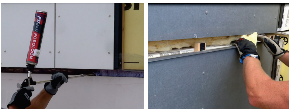
Figure 4.25 Joints between elements were filled with PUR foam (left) and mineral wool bands to avoid thermal bridges and minimise the convection (2017).
