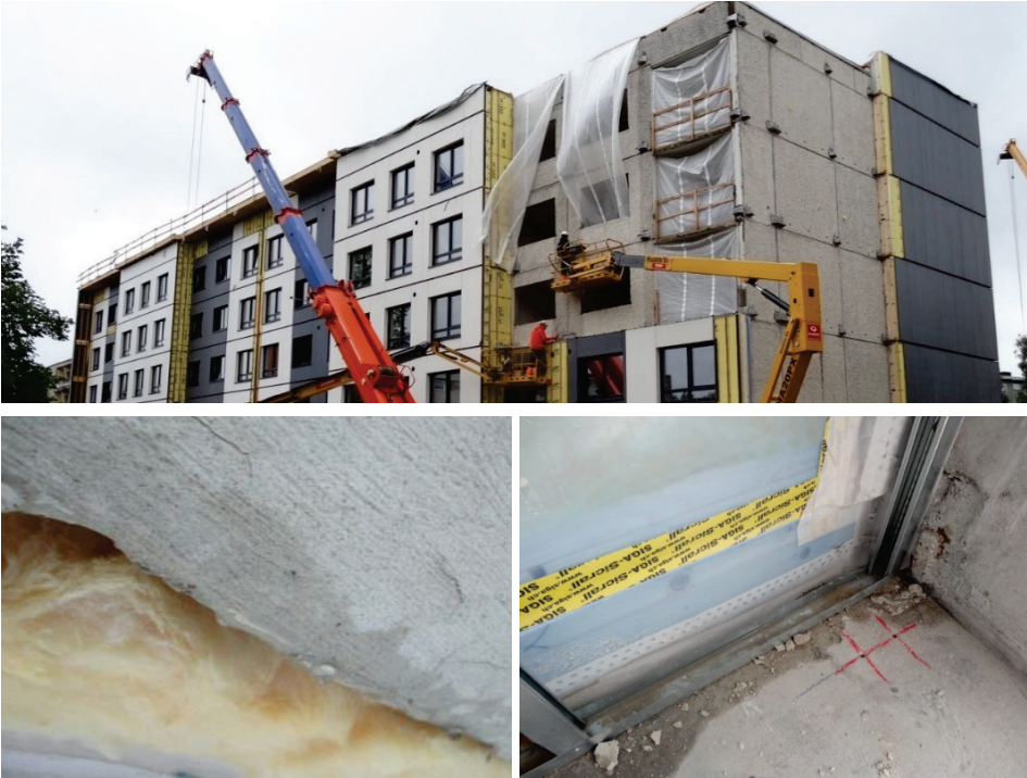
Figure 4.30 Installation of prefabricated insulation elements with insufficient moisture protection (top). Rainwater has flowed inside the element and between the element and the original PCLP wall (bottom) (2017).
