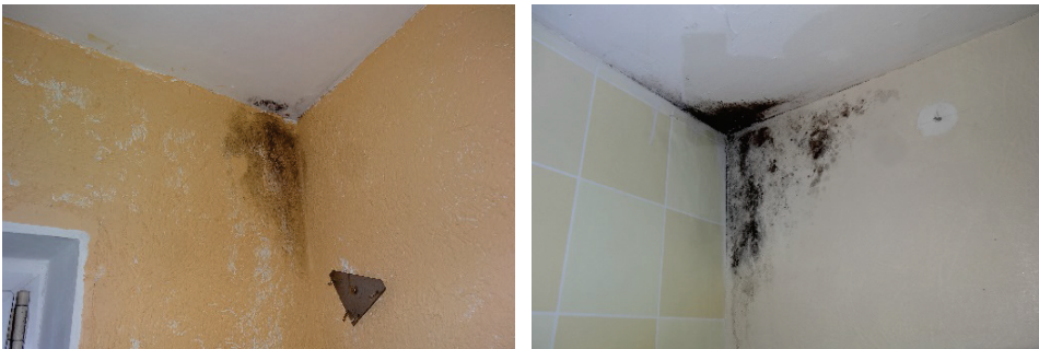
Figure 3.3 Mould grows on the surface of the connection of the external wall, internal wall and intermediate floor of the pilot building (2015).
