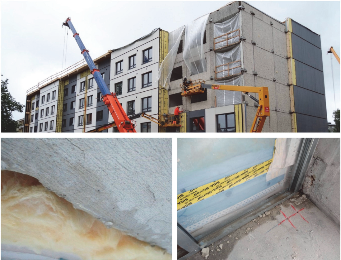
Figure 3. Installation of prefabricated facade insulation elements with insufficient moisture protection (top). Rainwater has flowed inside the element and between the element and the old wall (bottom).
