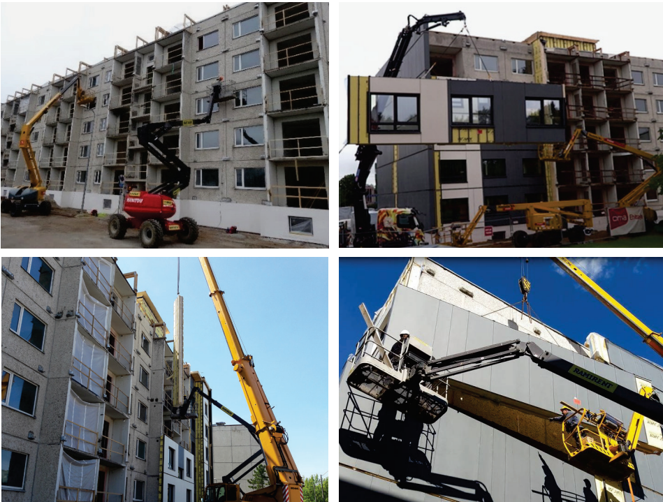
Figure 4.28 Open loggias are ready for prefabricated elements to be installed (top left). Lifting of a vertical wall element with embedded ventilation ducts (bottom left). Installation of the prefabricated timber frame insulation elements on the pilot building (right) (2017).
