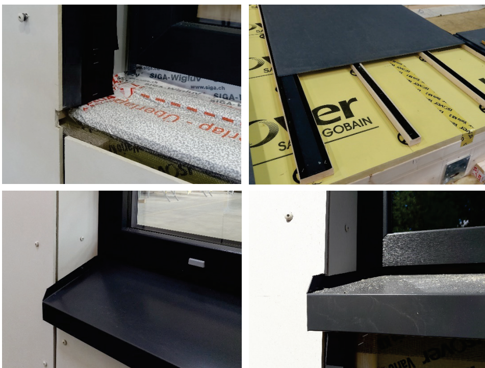
Figure 4.23 EPDM sealing and protecting steel strip on the window side (top left) and on the battens of the ventilated air gap (top right). Initially designed drip mould (bottom left) and revised final solution (bottom right) (2017).
