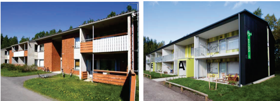
Figure 2.5 E2ReBuild demonstration project in Oulu, Finland. New insulation installed on facades, roof and ground floor slab and new technical appliances (Heim et al. 2014).
