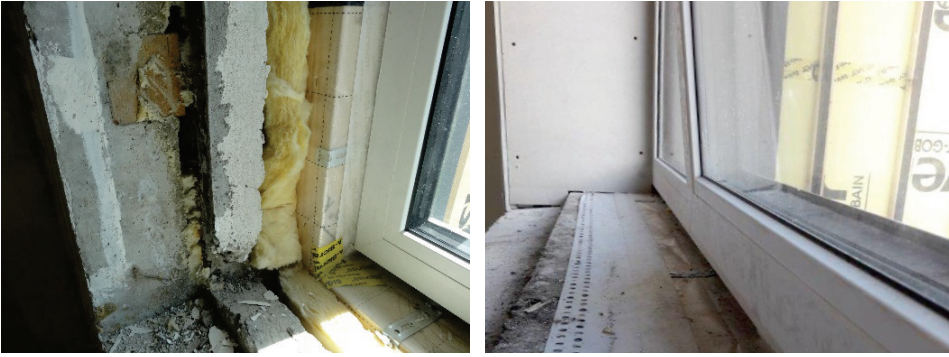
Figure 4.27 Old window block is removed (left). New window block in the prefabricated element and airtight sealing around the sides of the window opening (right) (2017).
