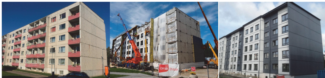
Figure 1. Overview of the building in 2015 before (left), in summer 2017 during (middle), and in autumn 2017 after (right) the nZEB renovation with prefabricated timber frame insulation elements.
