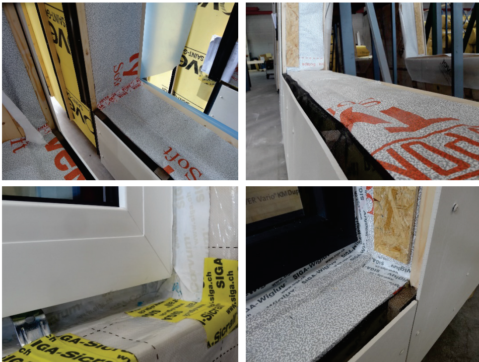
Figure 4.22 Wall elements are prepared for the installation of windows at the factory (above). Continuous sealing around installed window frames from inside (bottom left) and outside (bottom right) (2017).
