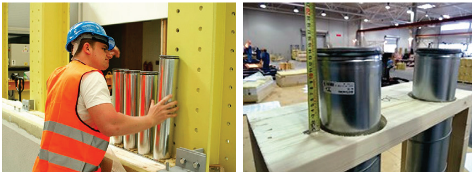
Figure 2.8 Modular pipe installation prototyping in the Czech Republic (left) and in Estonia (right) in the MORE-CONNECT project (2016).
