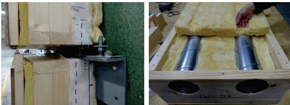
Figure 4.19 Prototyping of the prefabricated elements in 2016. Consideration of joint and hanging bracket (left). Trial of placing insulation around embedded ventilation ducts in the element (right).
