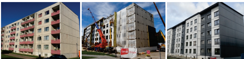
Figure 4.15 Overview of the pilot PCLP apartment building in 2015 before (left), in summer 2017 during (middle) and in autumn 2017 after (right) its deep energy renovation with prefabricated timber frame insulation elements. Photos from publication V.
