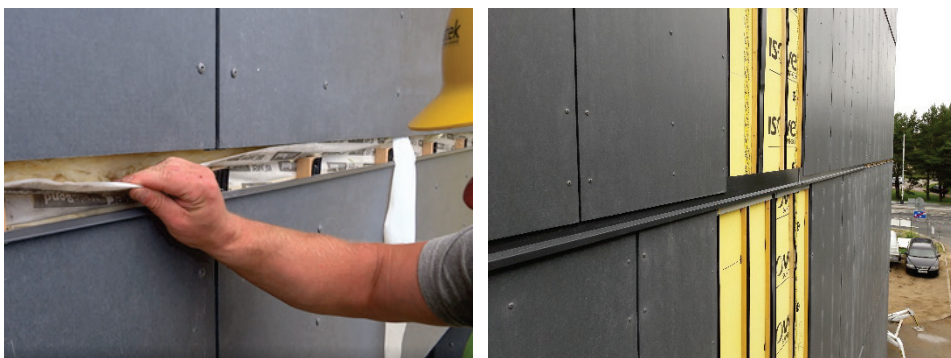
Figure 4.26 Self-adhesive sealant was used in the joints between the elements (left). Joints of facade boards were closed with steel strips and drip moulds preventing WDR overflow to the structure beneath (right) (2017).
