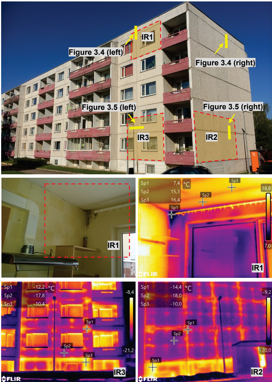
Figure 3.6 Measurement areas (top) and thermal bridges on the external walls (middle and bottom) before the nZEB renovation and installation of prefabricated elements (2015). Adapted from publication IV.
