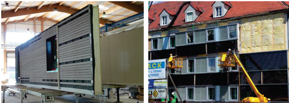
Figure 2.2 IEA ECBCS Annex 50 prefab elements production for the case study building in Switzerland (left) and assembly of the elements in the Austrian case study building (right) (Miloni et al. 2011).
