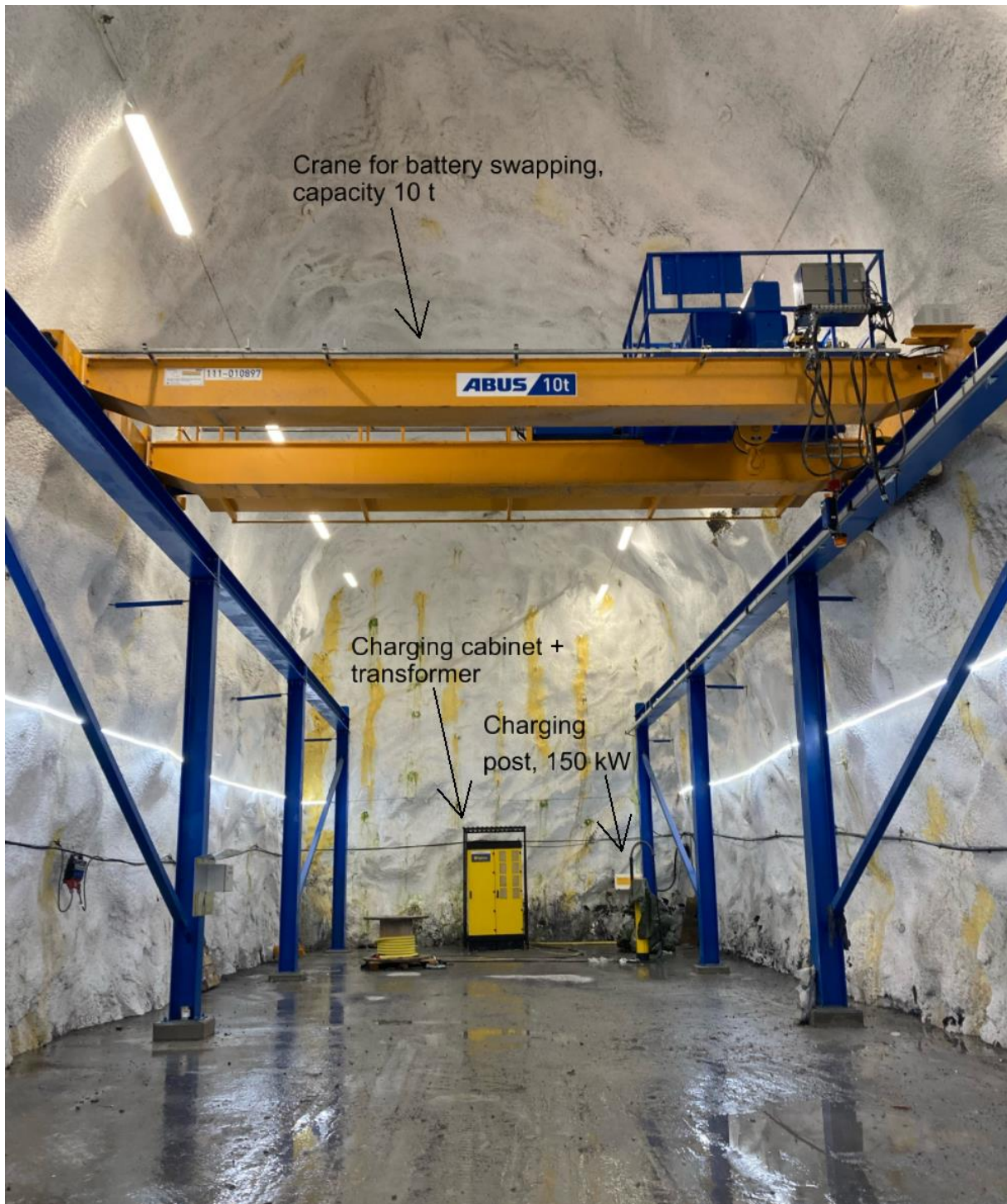
Figure 4.4 Battery Bay no. 1 on level 436 in Konsuln test mine
