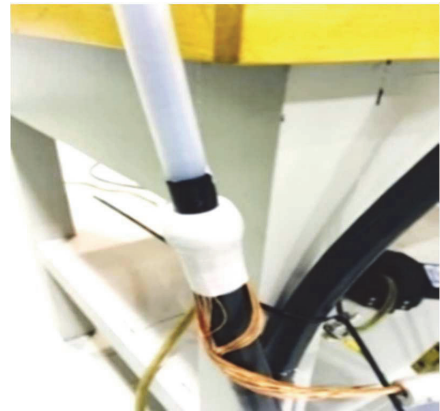
Fig. 3. 11 kV XLPE cable with defect by removing stress cone at the terminal for surface discharge.
