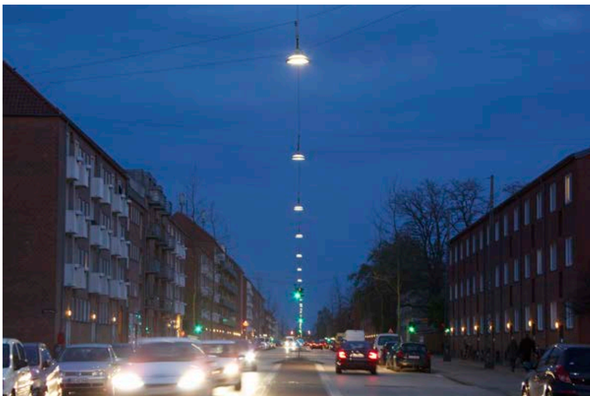
Figure 1. LED-based catenary luminaires in Copenhagen.
